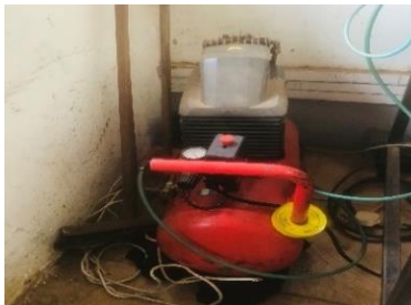
Picture17: The broken-down compressor that came with the machines which the team said was much better than the locally sourced.
