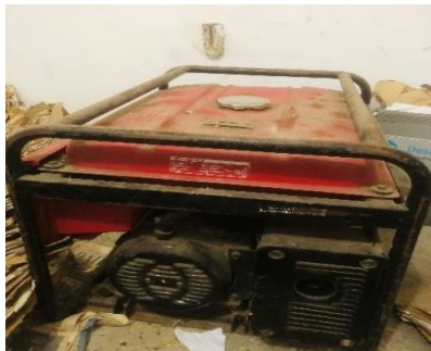
Picture12: One of the five generators in Tanzania
