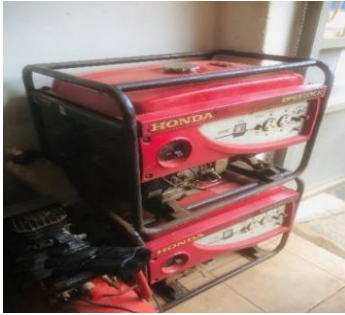
Picture15: The two generators for the Police in Uganda
